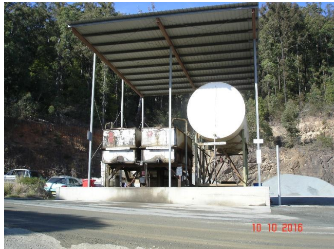
Aboveground Storage Tanks within bunding compliant with AS 1940.
